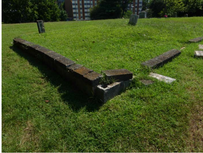
An example of a plot enclosure wall that requires repair of the curb capstone.
